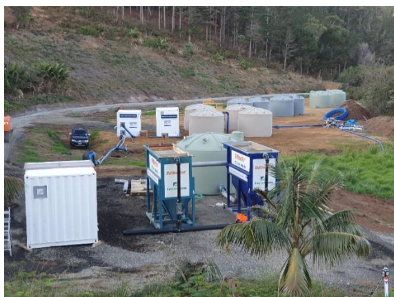
Back-up water supply: A tank farm and portable water treatment plant at Sweetwater last summer.
