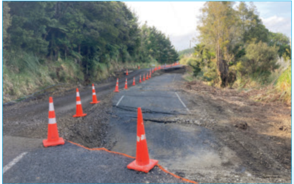
Repairs to two major slips on West Coast Road are expected to start early this year but may take some time. A detour remains in place for heavy vehicles at the Kohukohu slip.
